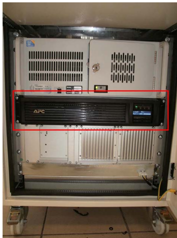
Fig. 3-20 PILOT V8 : Example of UPS
